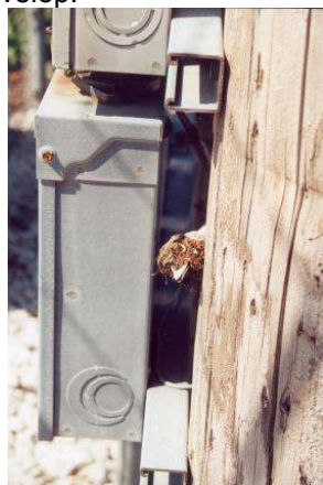
ChickEN found wedged behind an electrical box
