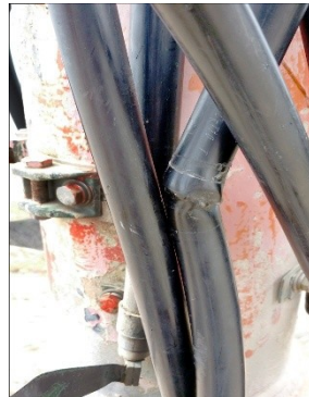
Closeup of kink on tower before removal.
