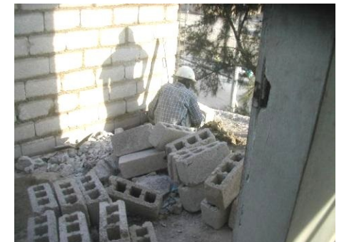
The mason working on the new room. The street is four floors down through the tree.
